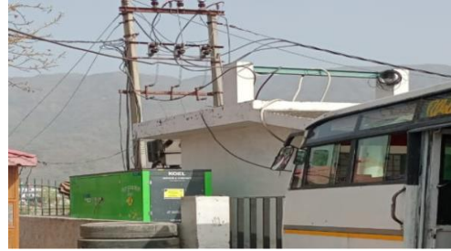
Transformer to be removed
